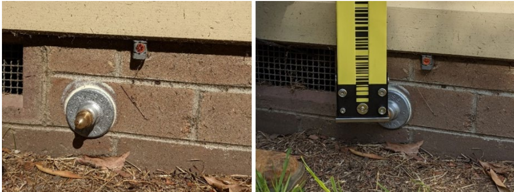
Figure 11: Levelling point glued just below the building mark reflector for OPL (including invar staff on right).
